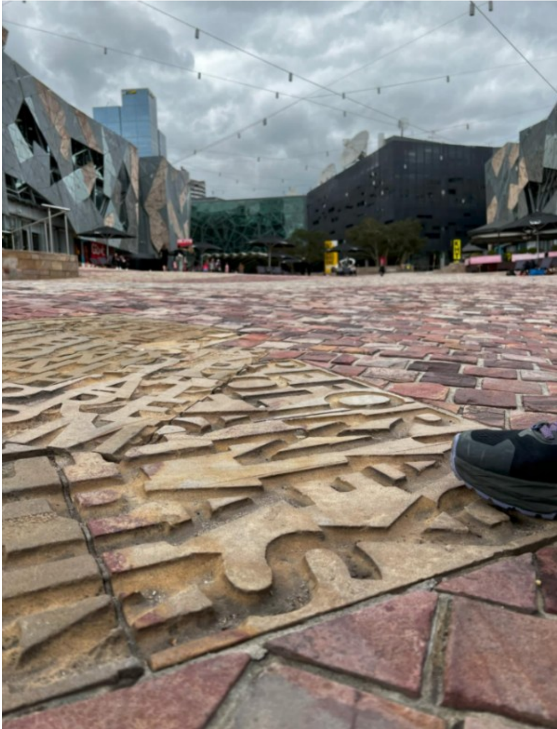
Figure 121: This rough surface installed in Melbourne, Australia would not be compliant with accessibility standards in the City of Guelph (Mark Steele, 2023)
